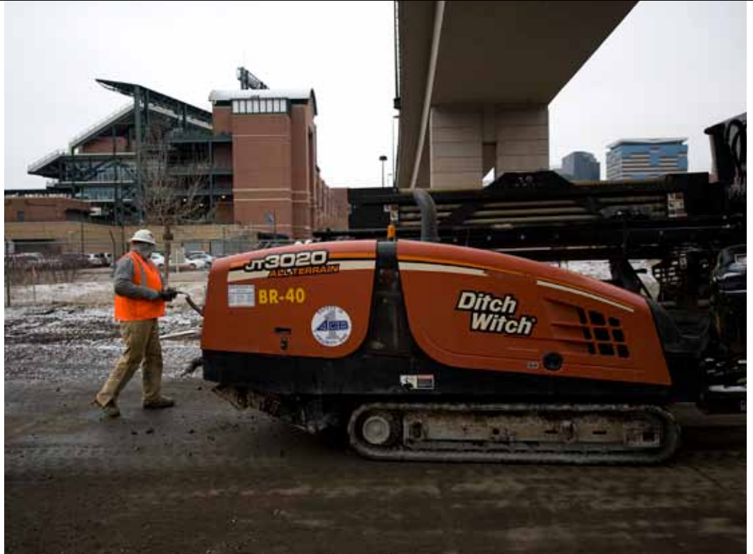
Construction worker starts the relocation of a major fiber optic cable for RTD's East commuter rail line to Denver International Airport.
